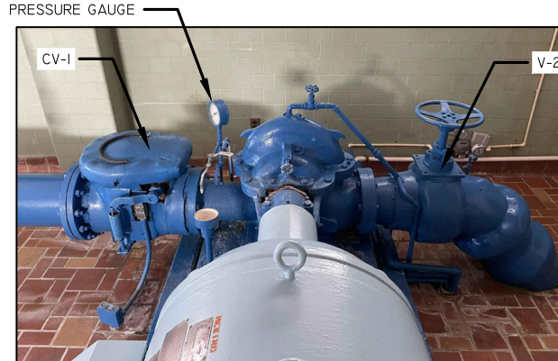
EXISTING PUMP CONFIGURATION FACING NORTH WALL
