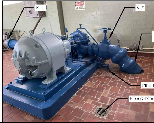
EXISTING PUMP AND MOTOR FACING NORTHWEST
