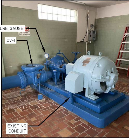
EXISTING PUMP AND MOTOR FACING NORTHEAST CORNER
